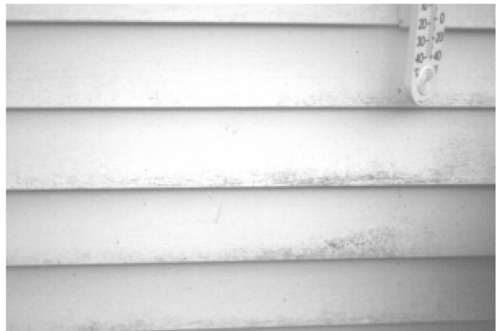
Figure 1. Mildew on side of house.
